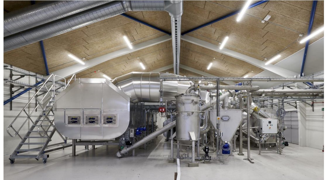
HECLA® Setores 1.000 at Fårevejle Wastewater Treatment Plant
